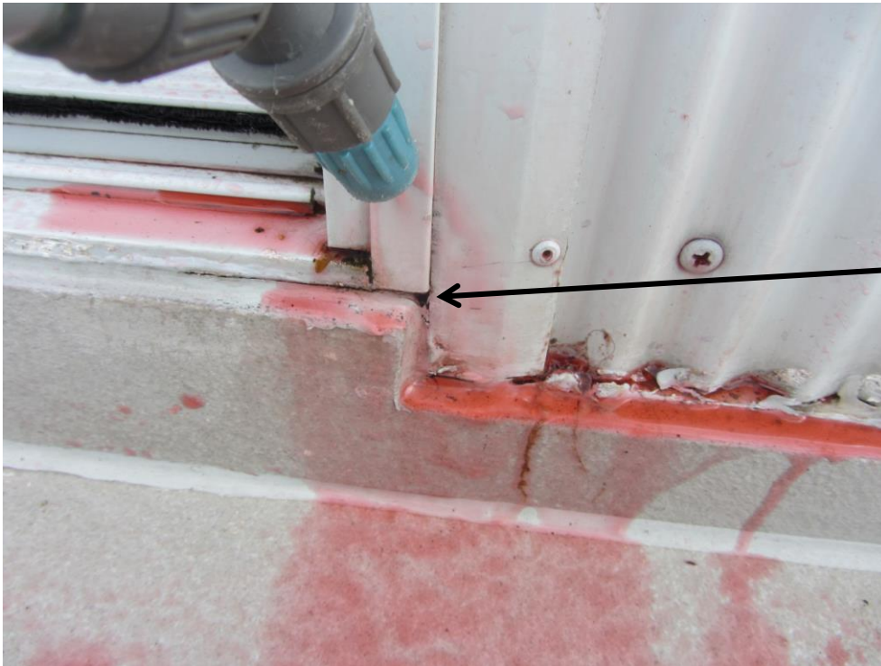
Photo 3. Test 2 in progress. The small gap in the caulking can be seen here.
