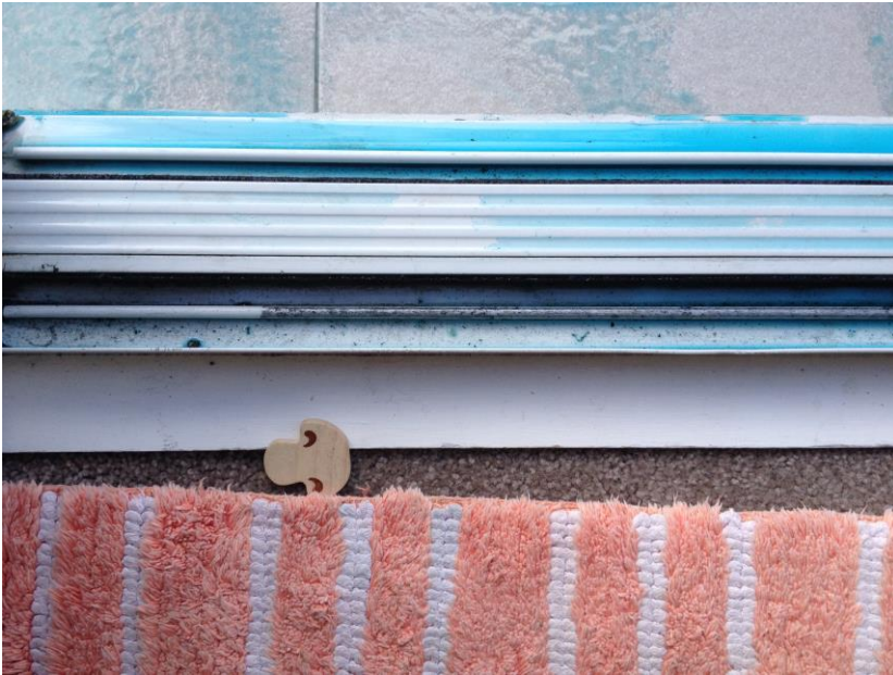
Photo 6. Water has seeped away through the base of the frame.
